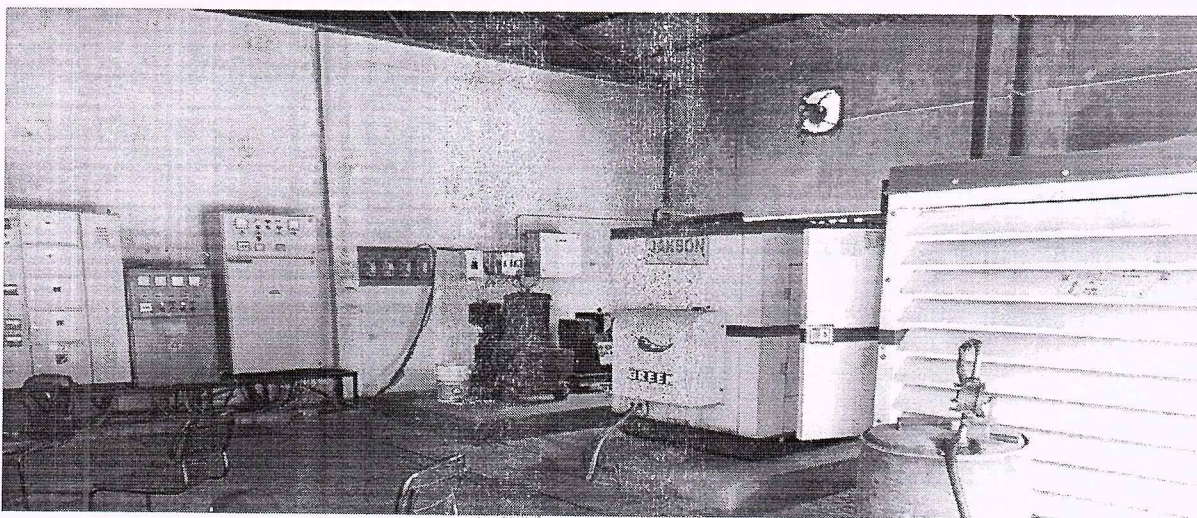
Electricity Generator Room
